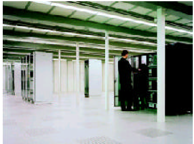
mTrack ASP Data Center
